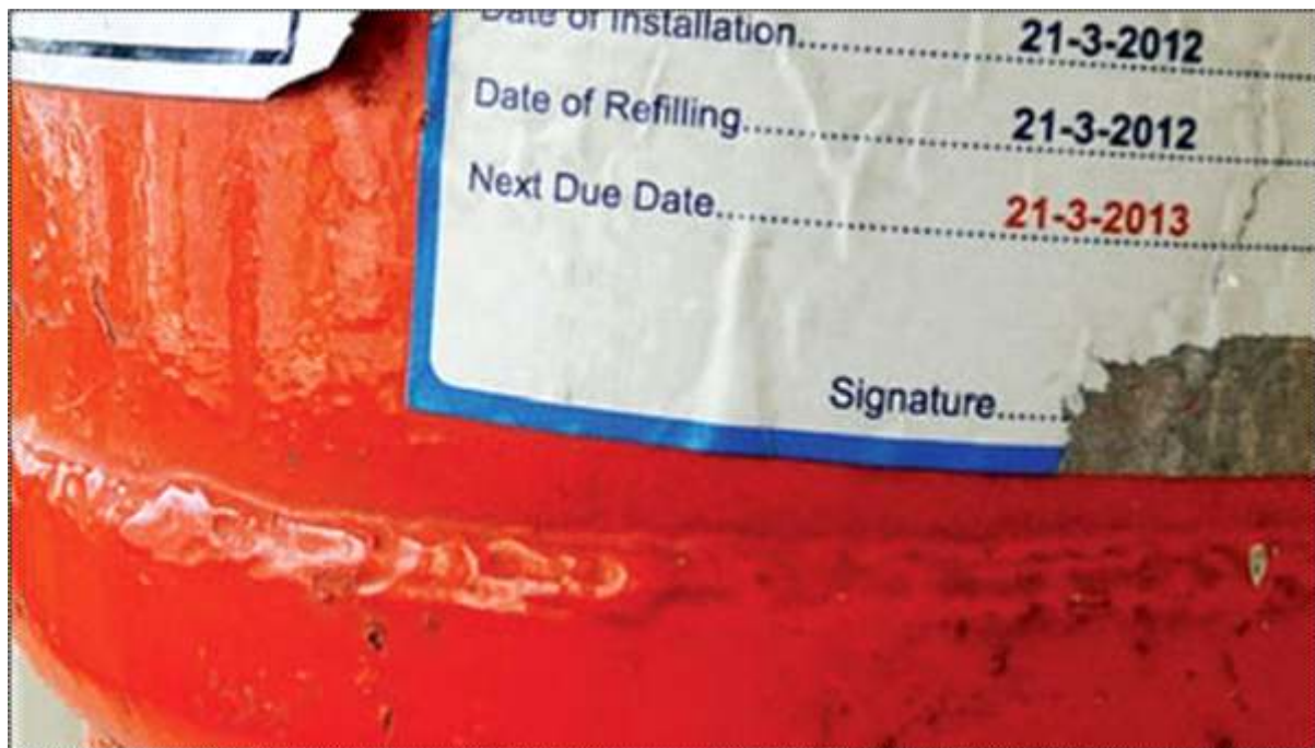
Fig 4.4.1.3 Know the refill date on the fire extinguisher
